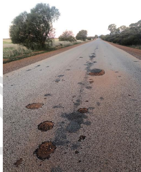
(L) This Image taken on 30 th June. These potholes have now been filled.
