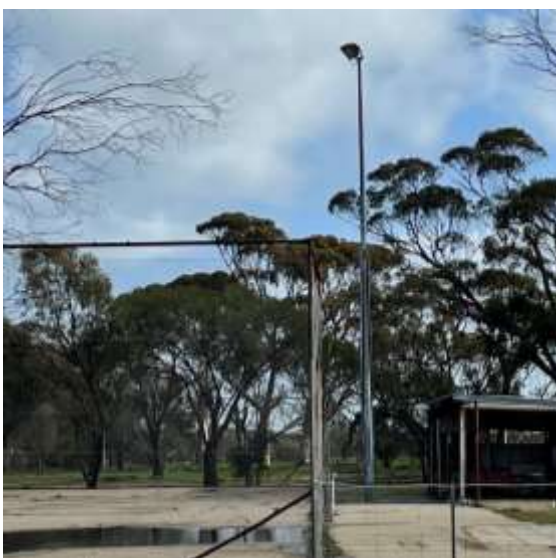
Tennis court lighting
