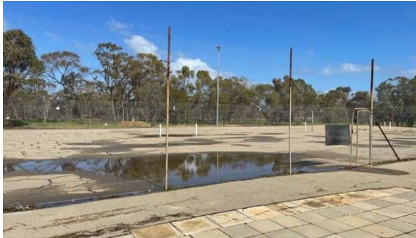
Tennis court surface in poor condition
