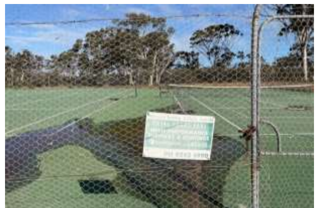
Surface uneven levels affecting drainage
