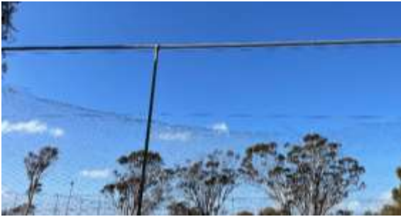
Fencing in poor condition
