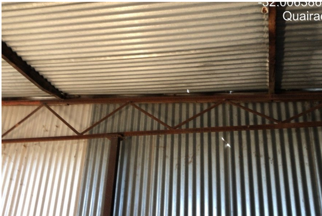
Deflecting Roof Sheeting
