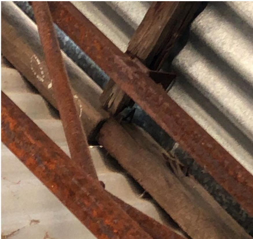
Damaged Barge/Rafter connection
